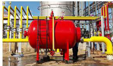
Foam Tank & Foam Equipment
